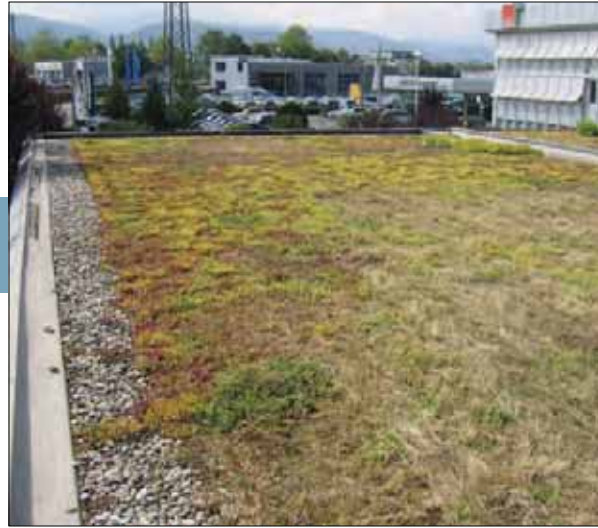
Figure 3.11 The integration of an extensive green roof atop the OMF would help trap runoff during storm events.
